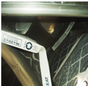
Example of moisture reducing frame strength of standard cardboard pleated filters. Filters have potential to blow out of racks and cause damage to air handler units
