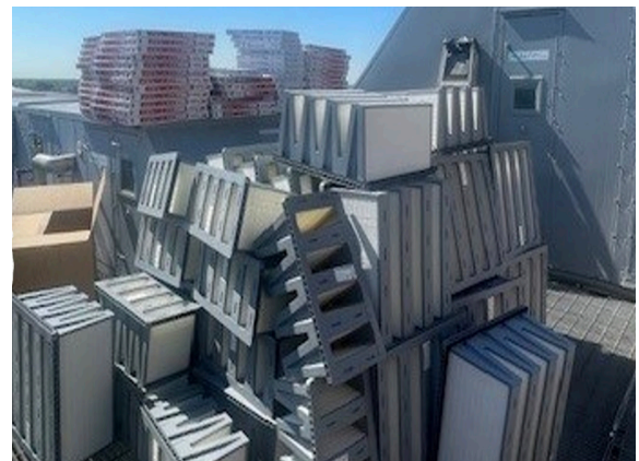
The MERV 16 V-Bank filters that were replaced
